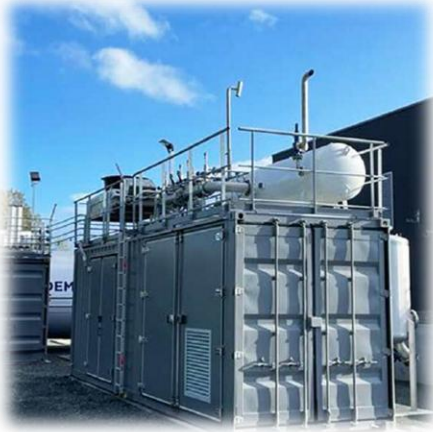
Biogenic CO2 collection, purification & liquefaction
