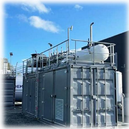
Biogenic CO2 collection, purification & liquefaction
