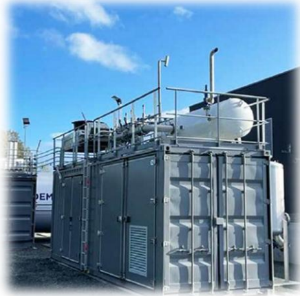
Biogenic CO2 collection, purification & liquefaction
